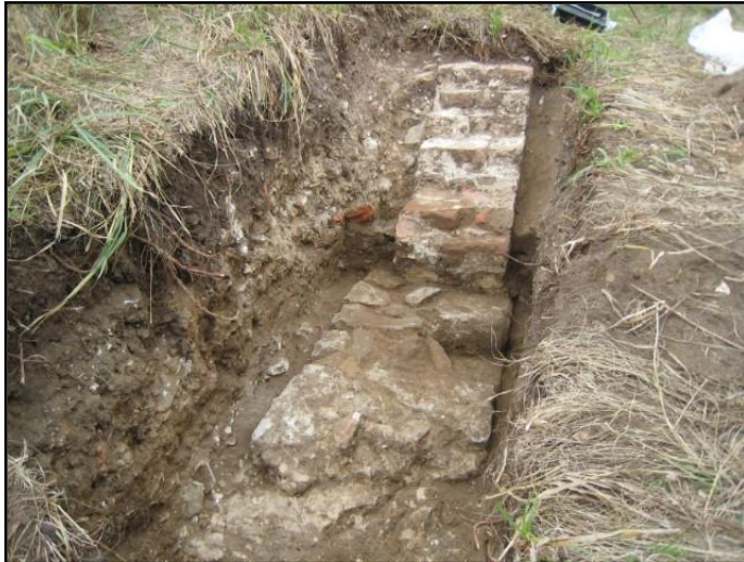
Fig 1 The southwest terrace retaining wall on its stone foundation close to the SW corner
